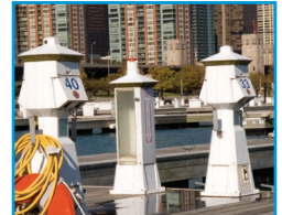
marine shore-power and dock lighting
